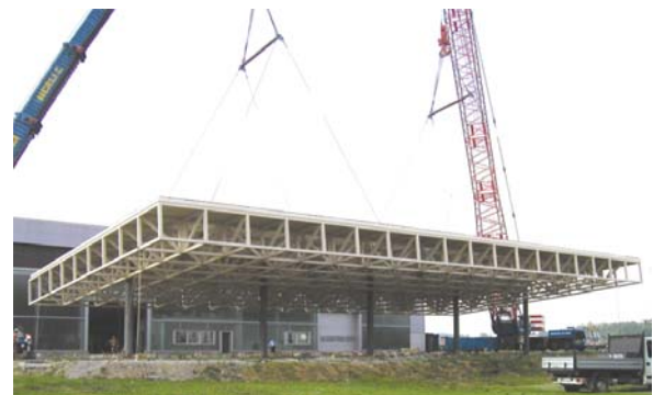
Figure 7: Lifting of a 1,000 m 2 spatial reticular cantilever roof in Bregnano, built on ground in a unique piece, with beams connected by CNP joints (2002)
