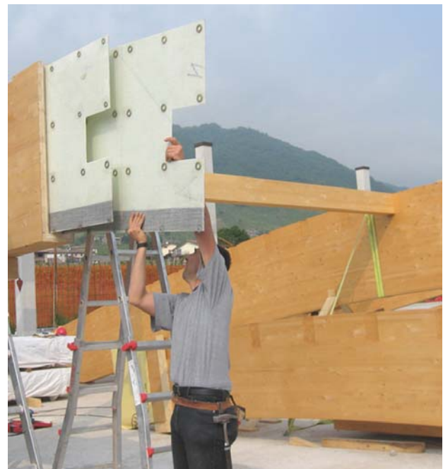
Figure 32: Placement of Giunto Italia ® with double GFRP inserts reinforced by carbon tapes
