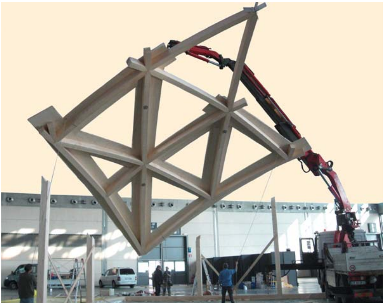
Figure 33: TechnoDomus exhibition, RiminiFiera, March 2009. Hypothesis of a space membrane in glulam and Polyever G800 woven rovings; for the multidirectional connections a multi-way Giunto Italia® in GFRP has been designed
